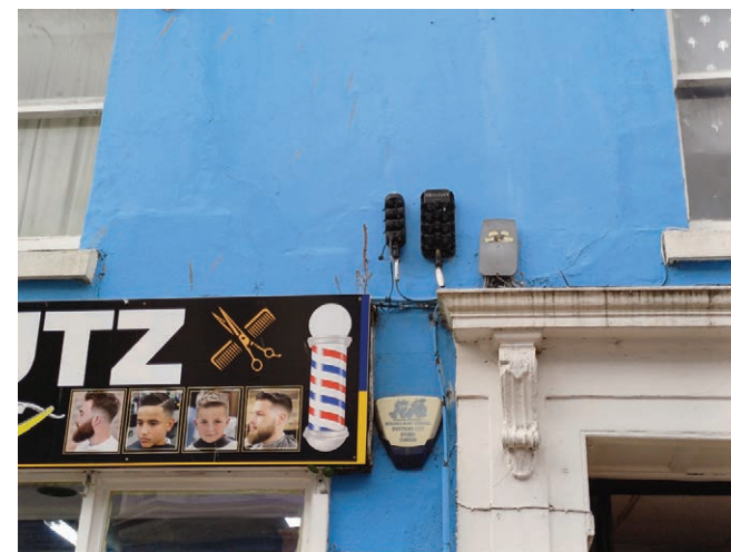
The accretion of wall-mounted services on this principal elevation detracts from the aesthetic interest of the host building and the wider streetscape.
