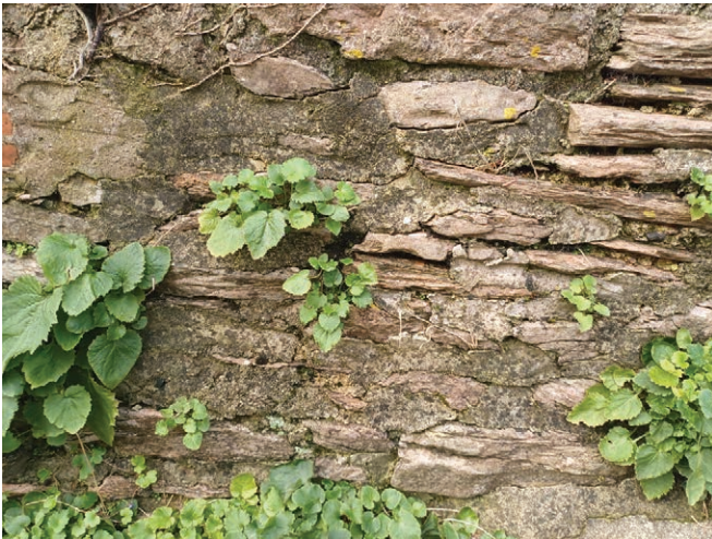
Detail of a boundary which has been repointed with non-breathable cementitious mortar and has extensive vegetation growth. A plant will typically root in mortar joints and force itself deeper as it grows, which can push the built fabric out of position and weaken the integrity of the wall.
