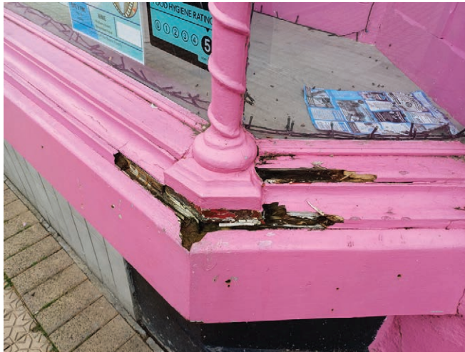
Rotting timber detracts from the aesthetic impact of this traditionally styled shopfront on Fore Street.
