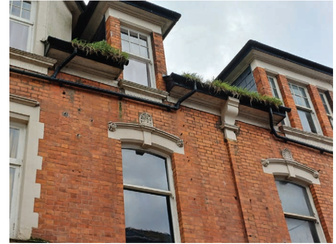
A gutter to a historic building on Fore Street, completely blocked with vegetation.
