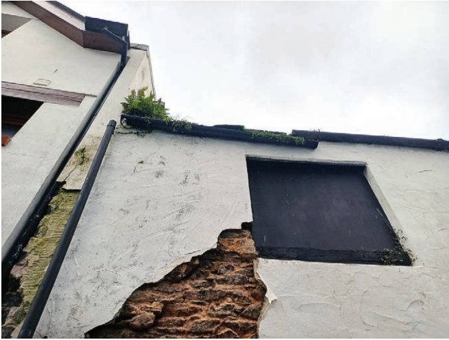
An example of a blocked and broken gutter and failing render to a property on Pump Street.
