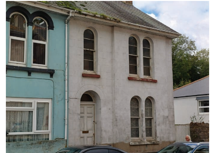
Deteriorating joinery to original windows at the end of this terrace on Bolton Street. The property is vacant.
