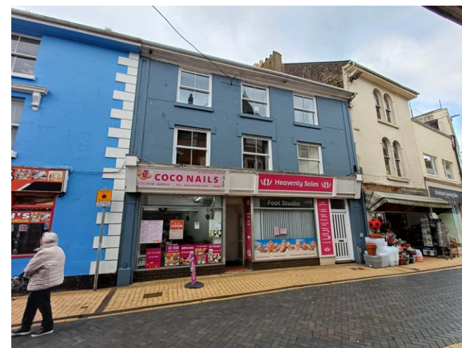
These shopfronts on Fore Street have been heavily modified through the replacement of the original window units with modern float glass and aluminium frames. Improvements might be made through the introduction of mullions and transoms and the rationalisation of advertising.
