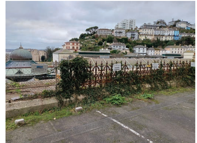
Lack of maintenance to the Grade II listed railings opposite St John's Church on Montpellier Road puts this important asset at risk.
