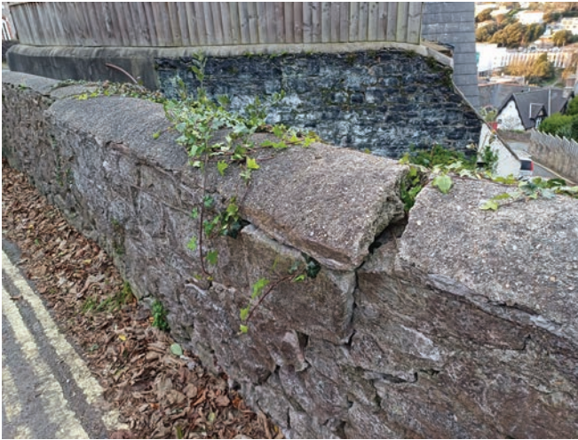
A deteriorating historic boundary wall on Vanehill Road.
