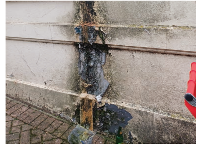
The bottom section of this downpipe is missing to a residential property on Braddons Hill Road West, which has resulted in substantial staining to the wall below.
