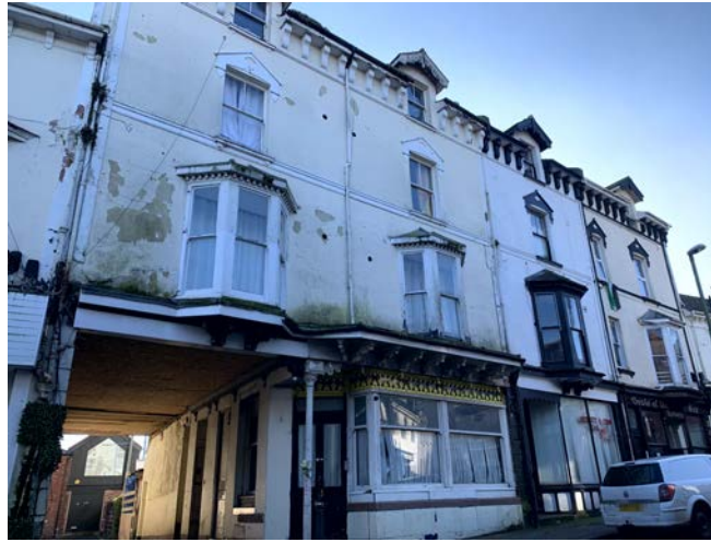
The former Crown and Anchor public house, now unoccupied and in a poor state of repair. The road through the carriage-arch is a thoroughfare through to Tower Road named after the pub, Crown and Anchor Way.
