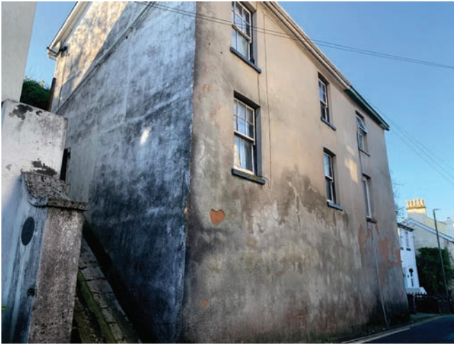
A house on Winner Street which has been externally rendered in concrete, leading to significant issues with dame which is causing areas of the render to fail.
