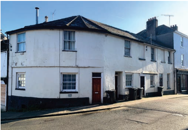
A listed house on the corner of Winner Street and Church Street which has been externally painted in a modern non-permeable paint leading to areas of cracking, bubbling and failure. The timber windows are also rotting in places.
