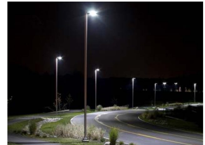
Low lux level lighting
