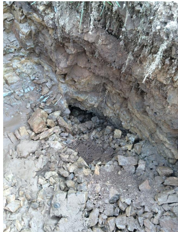
Plate 20 - TP9 showing the fissure in the base
