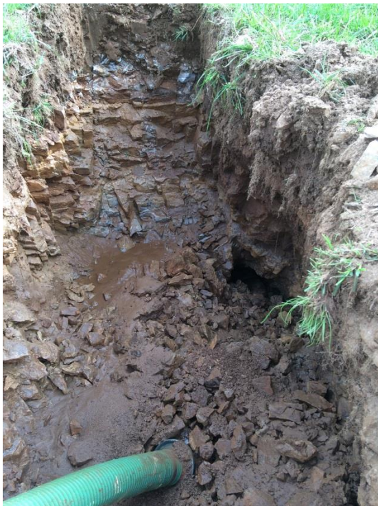
Plate 19 – TP9 showing the fissure in the base
