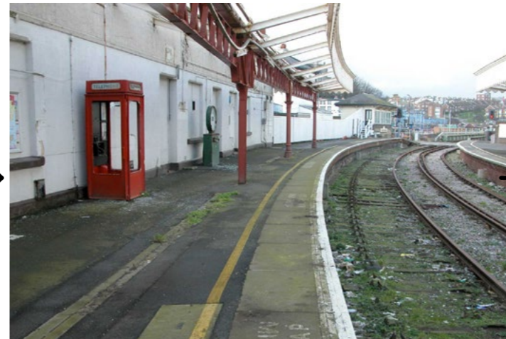
Falling into disrepair.
