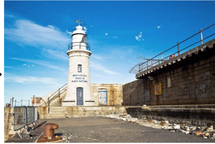
Falling into disrepair.
